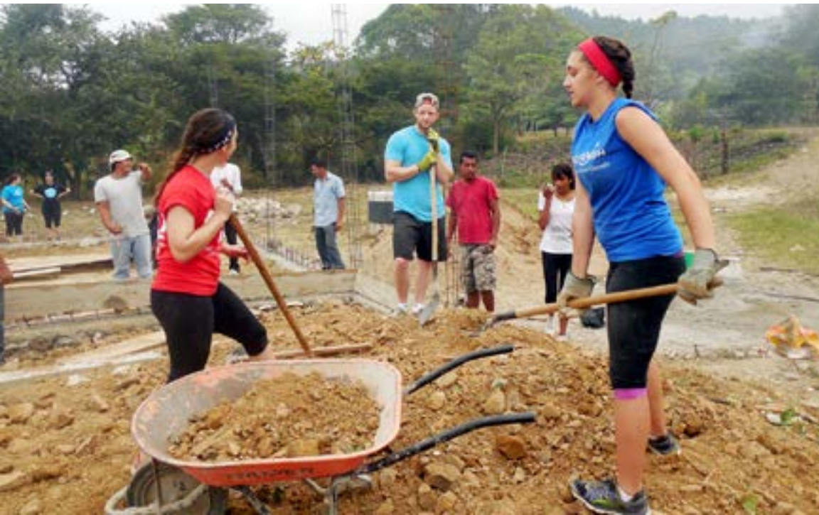
Carleton students in the Alternative Spring Break program digging the foundation for what will become a vocational training centre in Los Trozos, Honduras.
